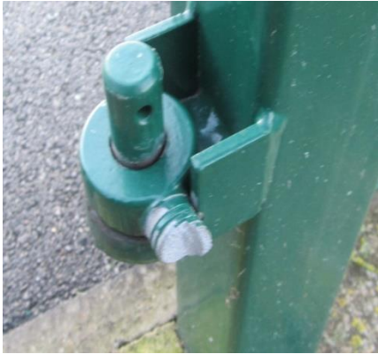
Photo 1: Gate post with 2 metal stops on lower hinge and part
